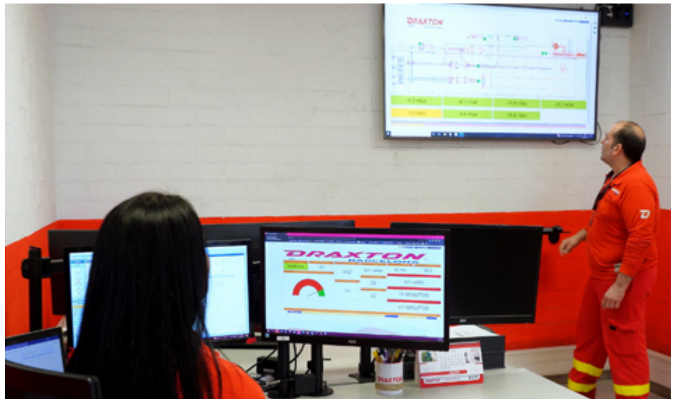
Draxton Barcelona's maintenance team use Monitizer | DISCOVER's dashboards that notify teams with alerts to support a proactive preventive maintenance program.
